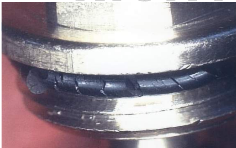
Fig. 19: Pre-assembled O-ring, which showed ozone cracks after several weeks due to the pre-stressing and ozone from the ambient air.
